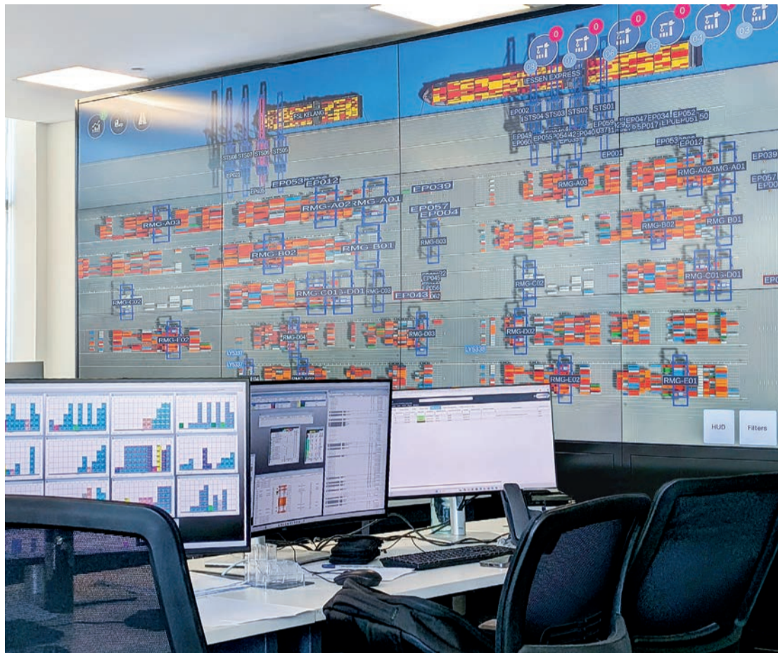
THE TWINBRIDGE in the control room. PHOTO: CAMCO
